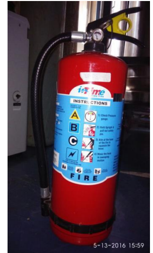
Fig: Fire extinguisher
