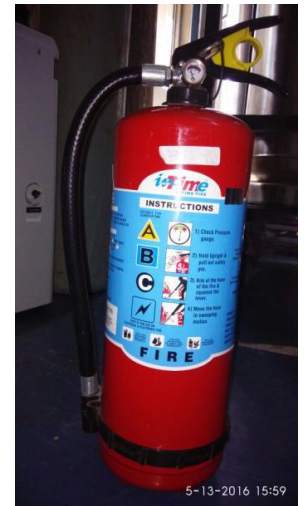
Fig: Fire extinguisher
